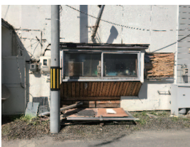
(c) 壁の崩落
