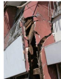
(e) 4本柱の折損
