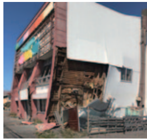
(c) 側面、壁の崩落
