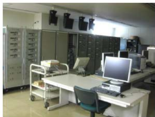
Loading Control Room
