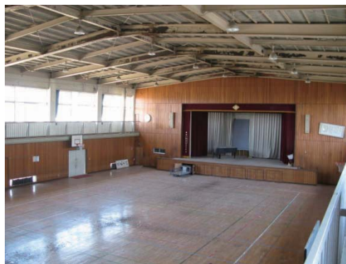
Photo 6.4-15 Peeling of paint of beams
