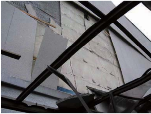
Photo 6.4-20 Falling of exterior finish components
