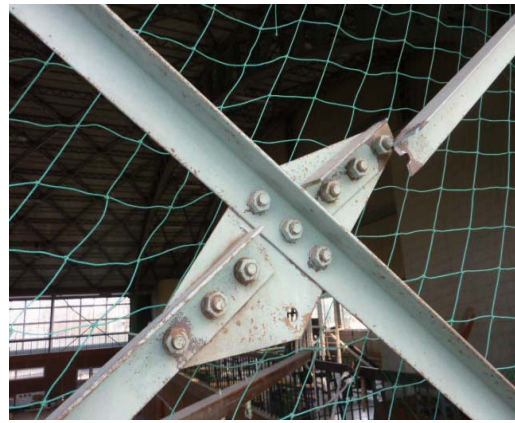
Photo 6.4-2 Net section fracture at bolt hole
