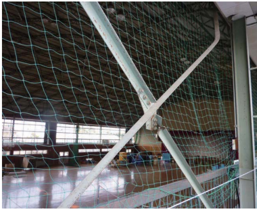
Photo 6.4-1 Buckling of brace
