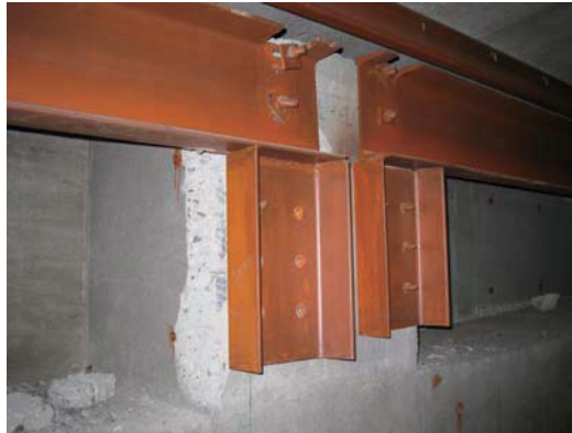
Photo 6.4-8 Pullout of hole-in anchors
