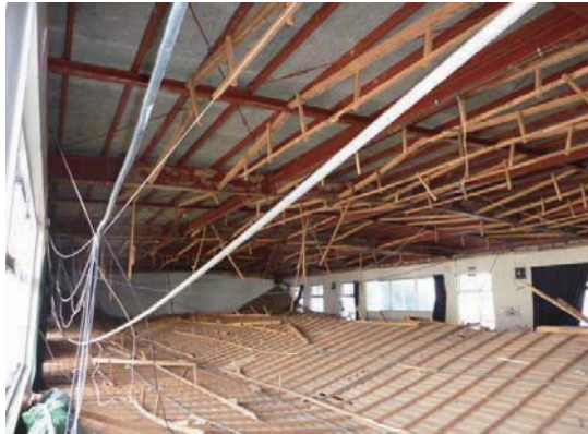
Photo 6.4-17 Dropping of extensive ceiling components
