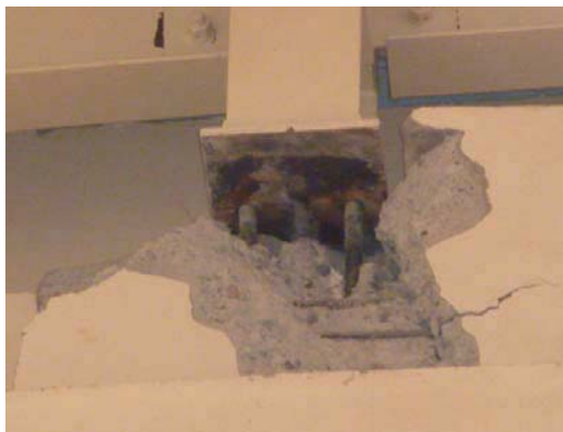
Photo 6.4-6 Spalling of concrete
