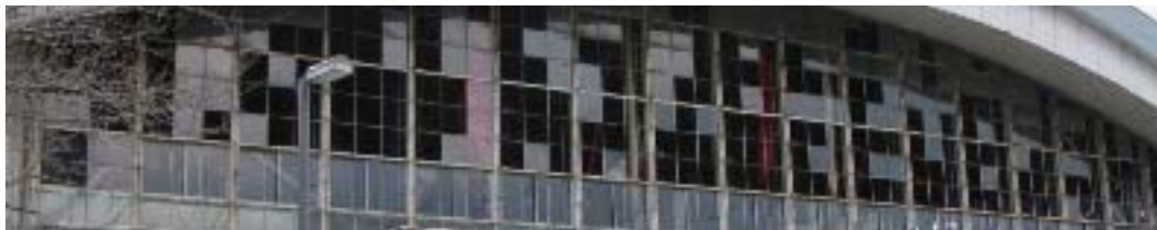
Photo 6.4-19 Breakage of windows
