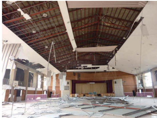
Photo 6.4-18 Dropping of extensive ceiling components
