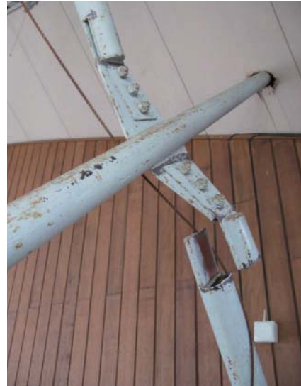
(b) Fracture at brace crossing
