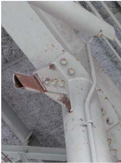
(a) Fracture at column top
