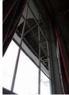
Photo 6.4-21 Falling of eave soffit
