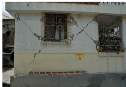
Masonry Shear wall Crack (Window)
