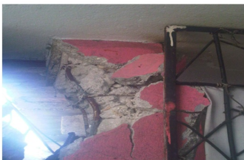
Concrete Column Rupture
