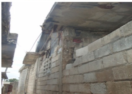
Wall out of plane Failure
