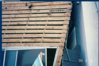
Narrow boards nailed to frame cannot resist lateral forces (1995 Kobe EQ)
