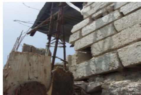
Partially disconnected wall
