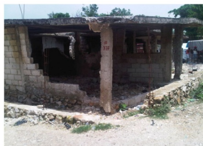
Masonry Shear wall Crack (X-Crack)
