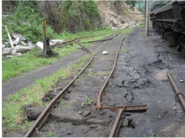
Rail track damaged and the train derailed
