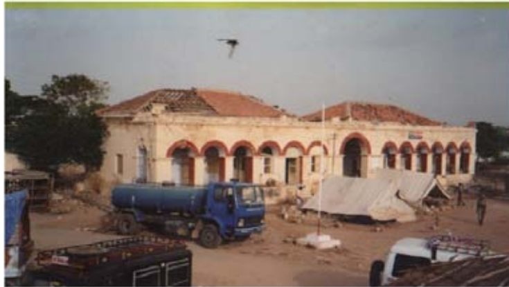
Damaged POLICE STATION BUILDING AT RAPAR
