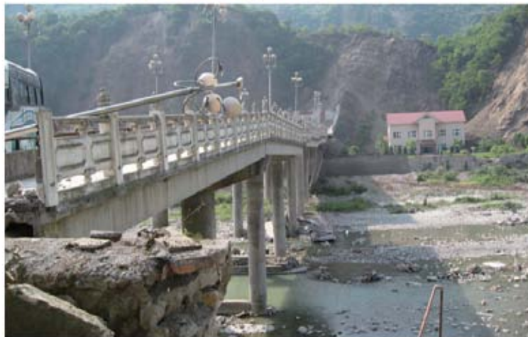
The damaged bridge in Beichuan town
