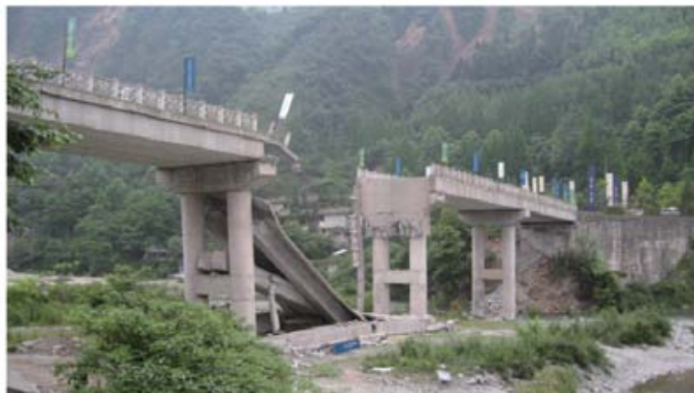
The Collapsed bridge in Beichuan town
