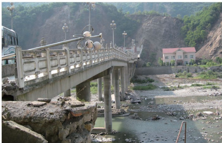
The damaged bridge in Beichuan town
