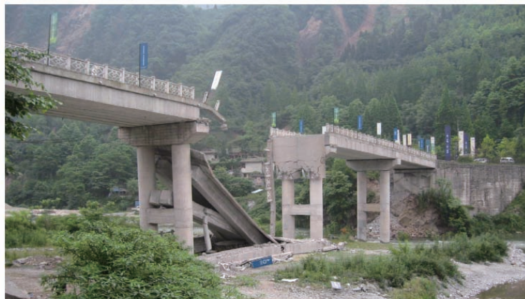
The Collapsed bridge in Beichuan town
