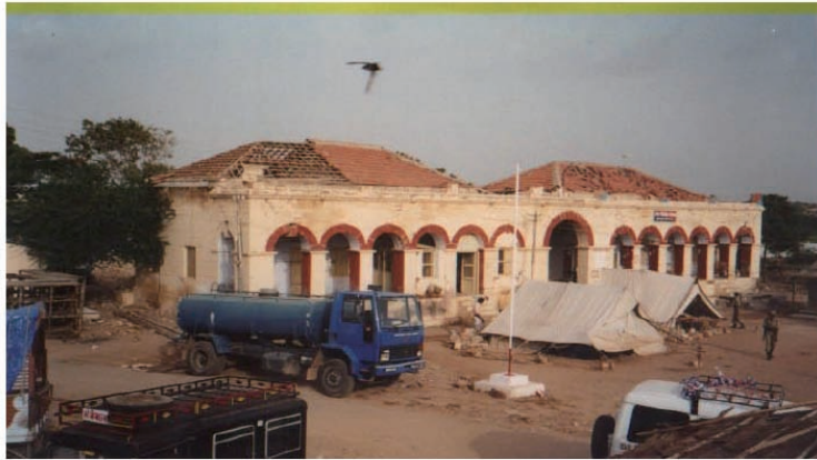
Damaged POLICE STATION BUILDING AT RAPAR
