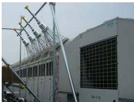
Figure 2.2.1-5. Static outlet air sampling device
